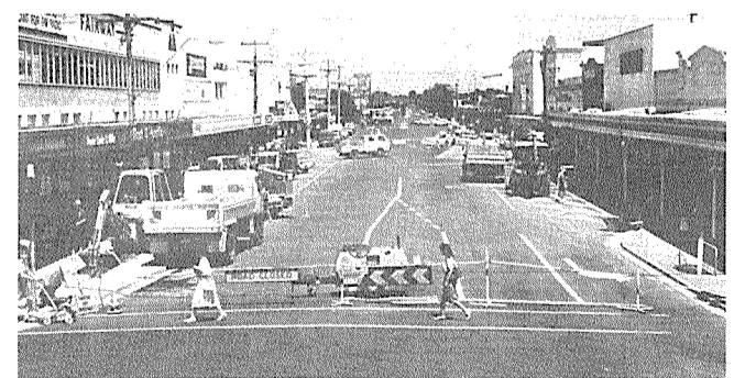
▲ Shepparton's Maude Street when work began to convert it to a mall - it was opened as a mall in 1986
